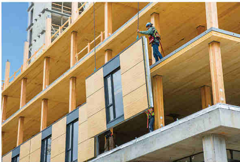
The prefabricated facade consists of steel stud framing with exterior sheathing, insulation and Trespa® Meteon® [distributed by ATS-Sales] for the rainscreen, attached with fibreglass 'Cascadia Clips' which significantly reduce thermal bridging compared to a more traditional metal girt cladding system.
